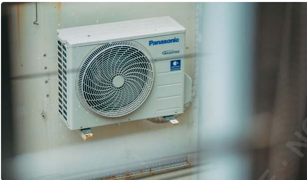
Mini-split condenser unit
