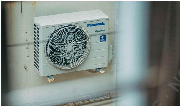
Mini-split condenser unit
