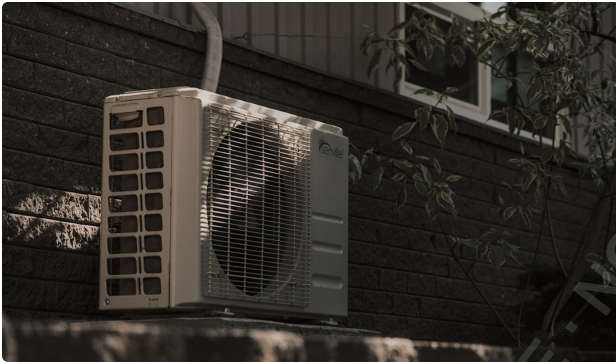
Heat pump condenser unit
