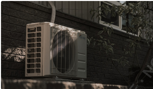
Heat pump condenser unit
