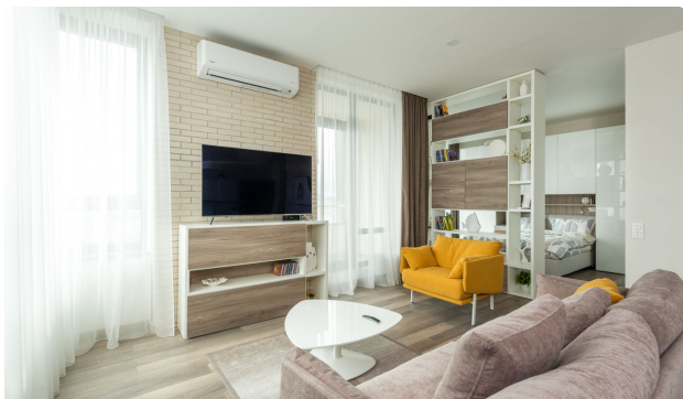
Wall-mounted mini-split AC unit
